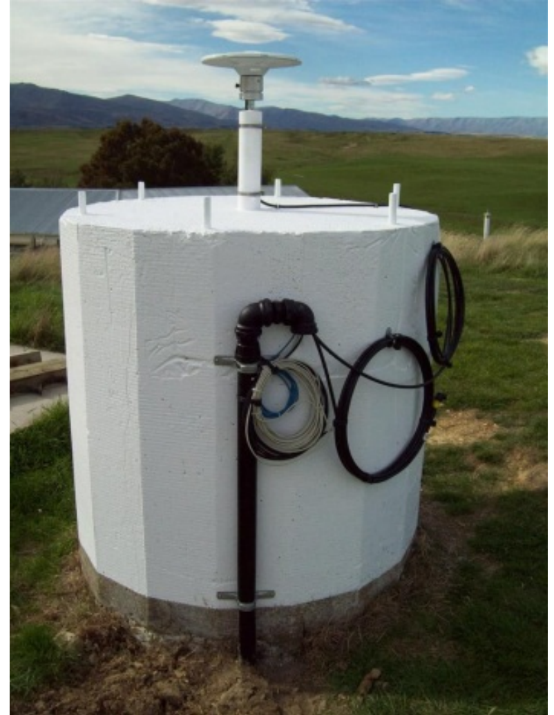
(right) GPS instrument on concrete pedestal with cabling
